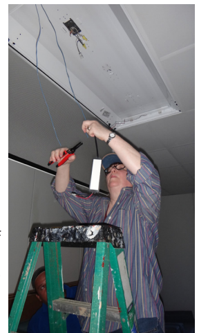
Lois Davidson of First Light Project installs the new LED lighting and ballasts.
